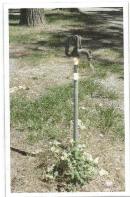
Frostless Hydrant in Park
