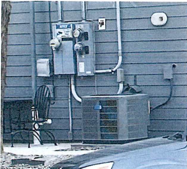
201 E. Main St. HVAC- NEW Unit
