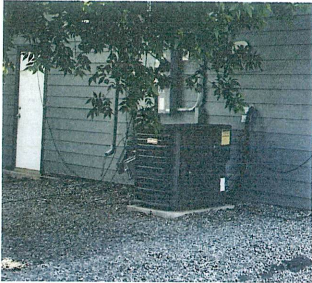
201 E. Main Street- HVAC -Old Unit
