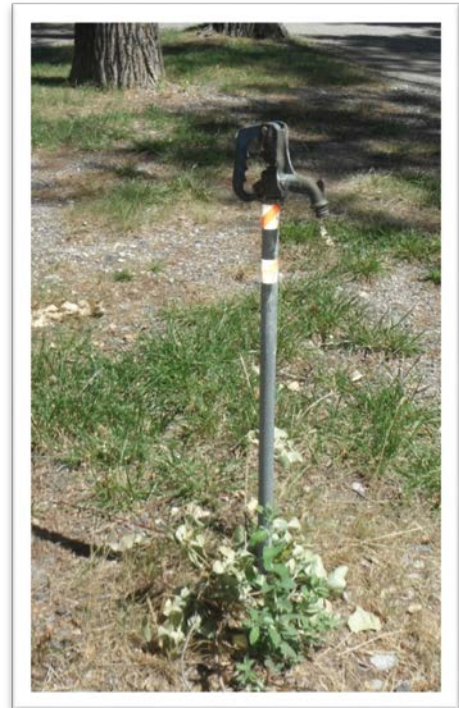
Frostless Hydrant in Park
