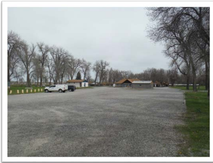
Existing Road Surface in the Park
