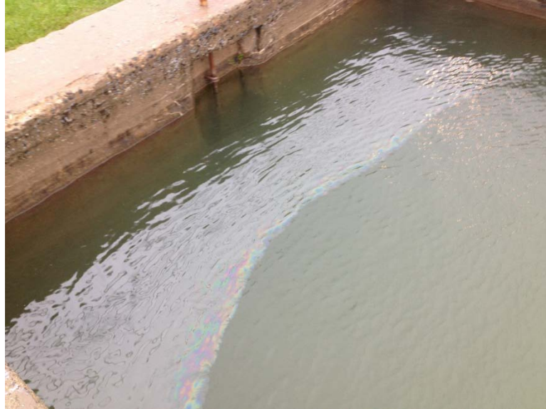
Figure 41: Diesel in sediment basins at Laurel WTP
