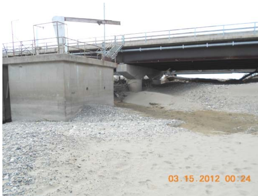
Figure 2: Original intake structure and sediment deposition, looking upstream at highway bridge
