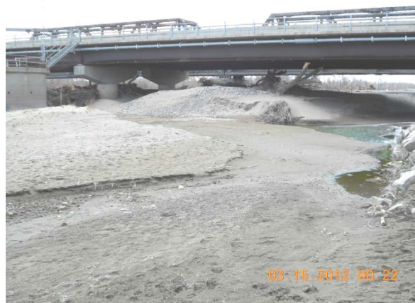
Figure 18: Sediment deposition beneath railroad and highway bridges. Looking upstream.
